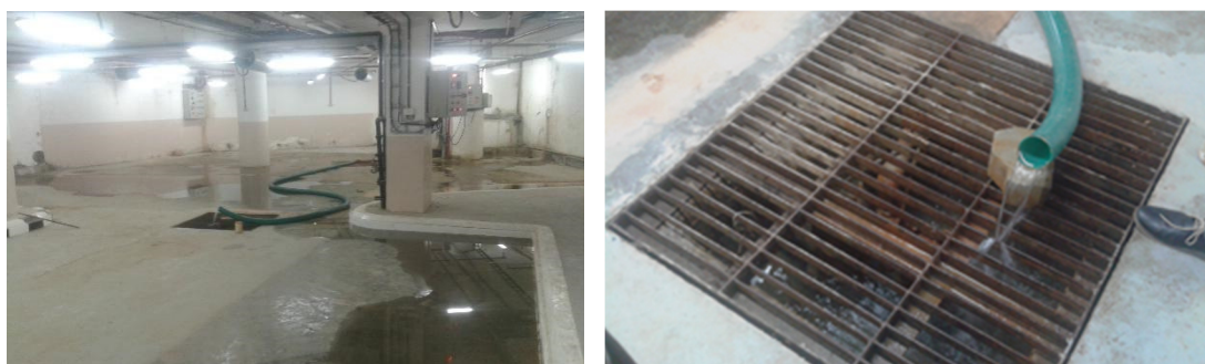
Water over-flowing from storage tanks
