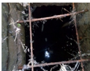
Water logged structure at RPS Infrastructure, Faridabad
